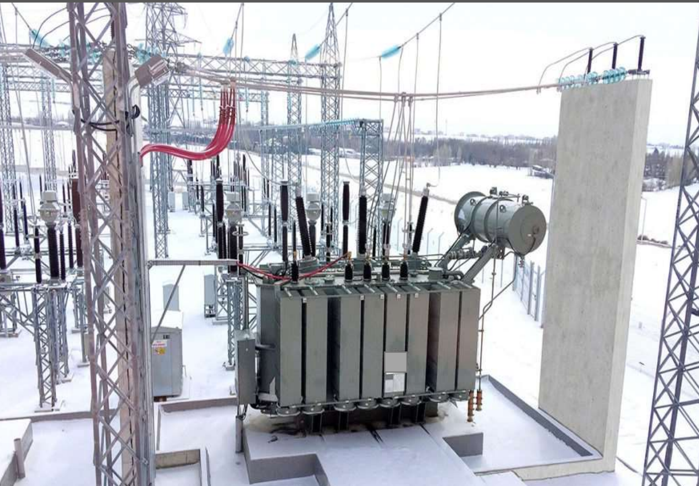
HV POWER TRANSFORMERS
