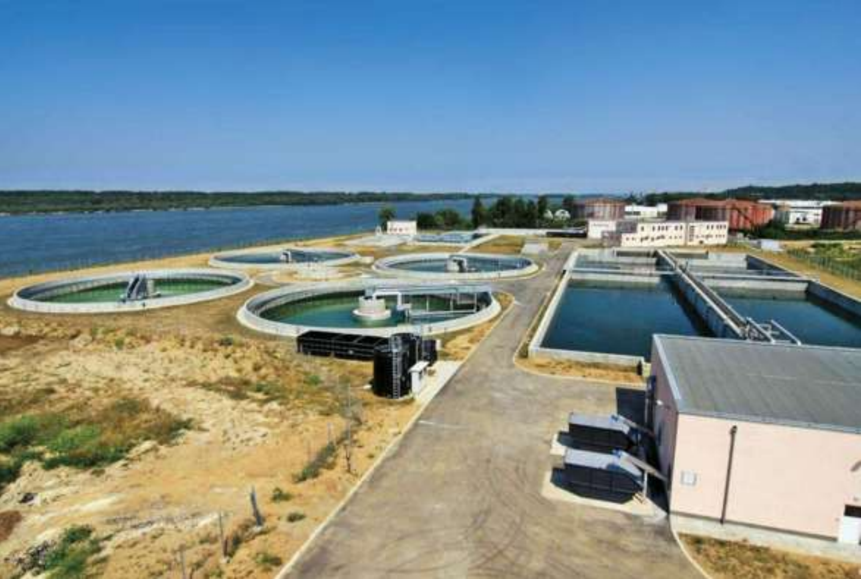
SATU MARE-ROMANIA WASTE WATER TREATMENT PLANT
