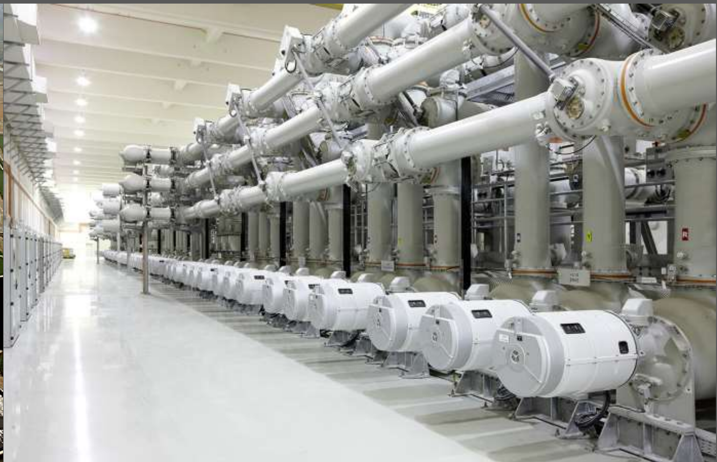
4 X 400 KV GIS SUBSTATIONS AMARA / IRAQ
