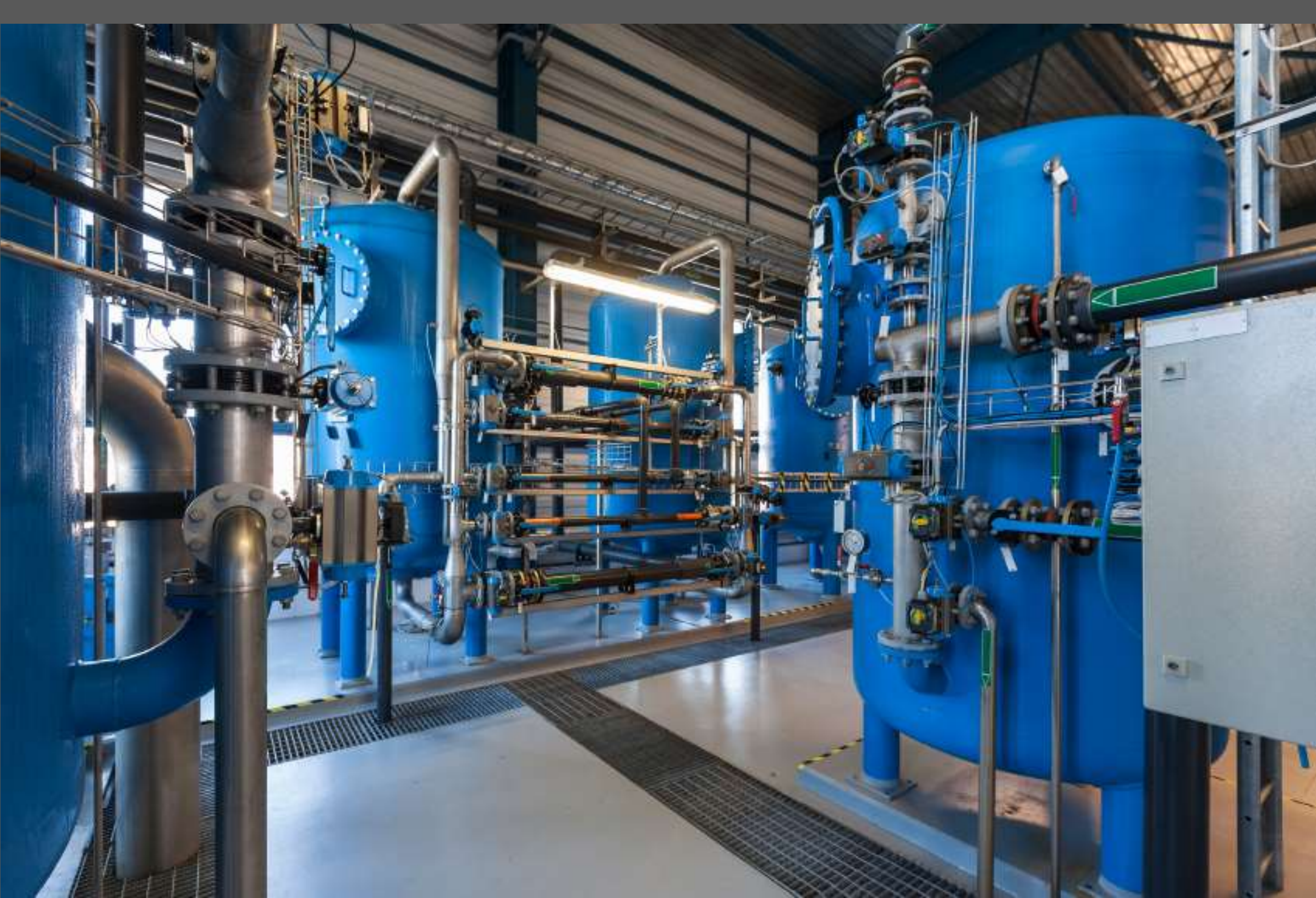
WATER PURIFICATION PLANTS
