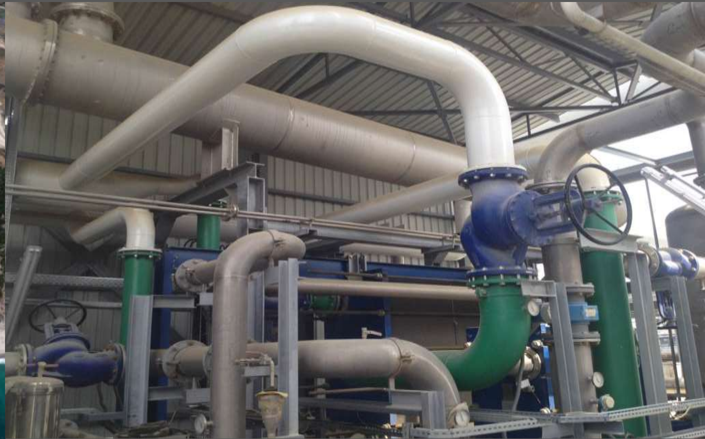
CO2 PLANT BAKU / AZERBAIJAN
