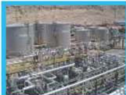
Co2 Plant - BAKU / AZERBAIJAN
