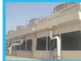
Cooling Towers - BAKU / AZERBAIJAN
