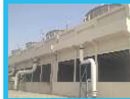
Cooling Towers - BAKU / AZERBAIJAN
